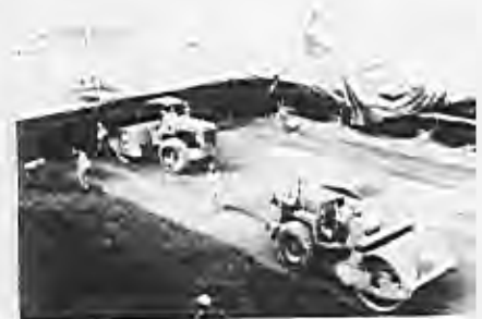
At Tucuruí, spreading of the rollcrete was carried out in one block while compaction was accomplished in another. Rolls of plastic were kept on site in case of rain.
