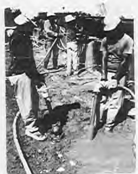
The jointing of the conventional concrete and the rollcrete was done by vibration.
