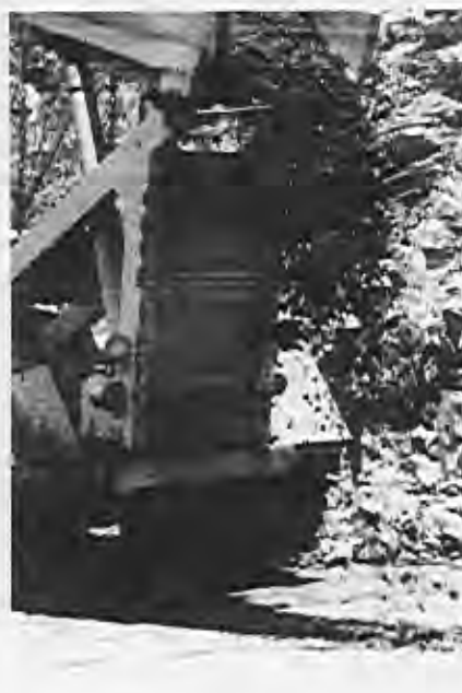
At the Tucuruí Dam project, the rollercrete was placed upon a thin layer of mortar.
