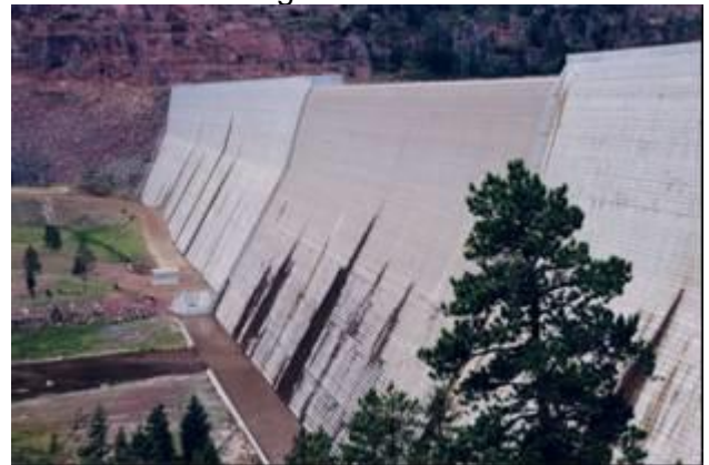
Figure 01- Cracks in the Upper Stillwater dam, resulting from thermal generation
