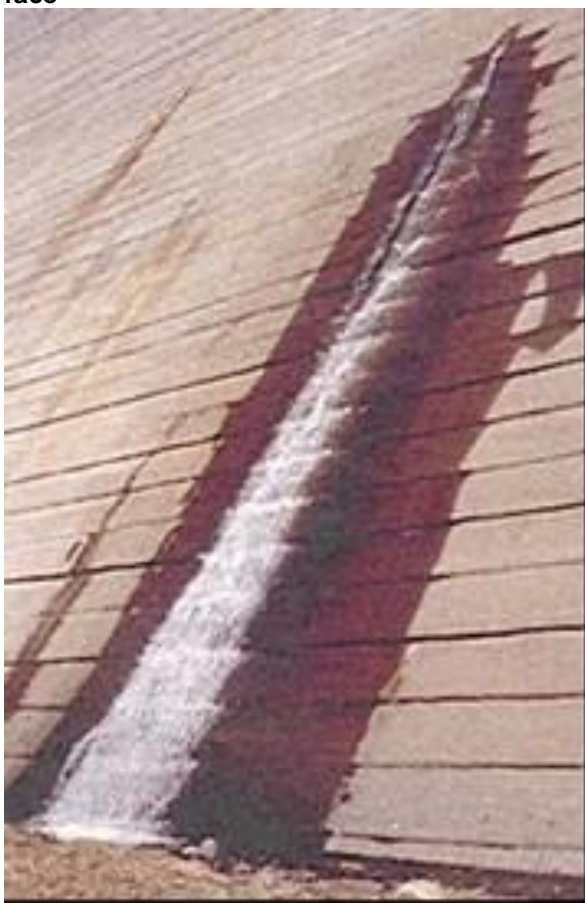
Figure 07- Cracks and leakage in Upper Stillwater [24,25]
